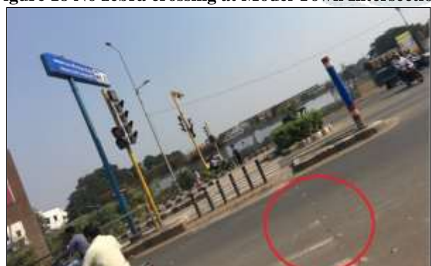
Figure 20 Improper Road markings at Dindoli intersection
