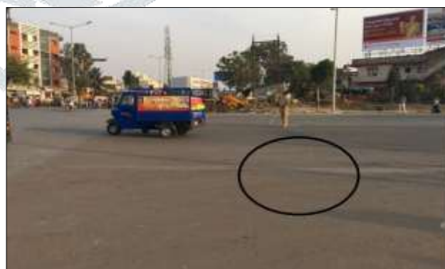
Figure 21 Improper Road markings at Dindoli intersection
